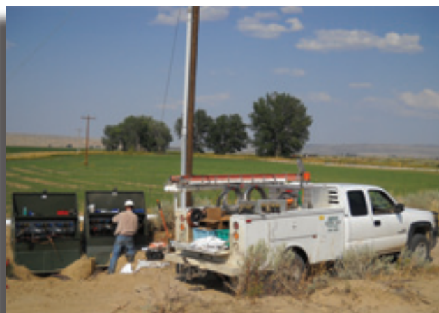
BEC Line Sub-Foreman, Lee Hauge, makes final connections of the underground feed to the Fish Hatchery.
