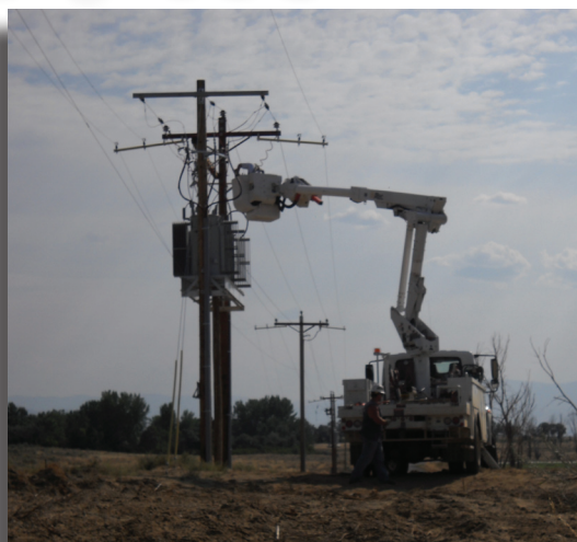
BEC Linemen, Eric Elton and Jason McDonald, install a new step down transformer during the Wyoming Conversion Project.
