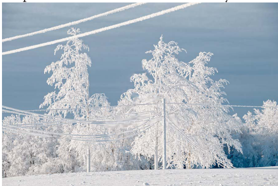
Snow load on distribution lines.
