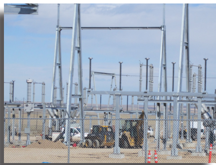
Northwestern Energy—230kV substation.
