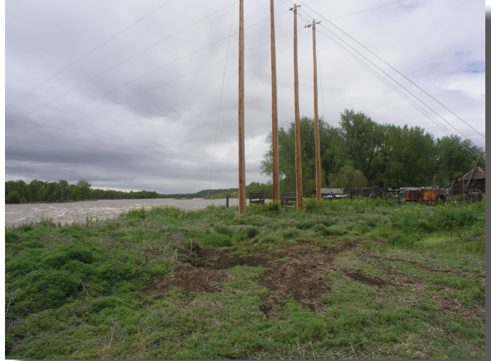
Yellowstone River bank 3 phase crossing moved 400 feet inland.
